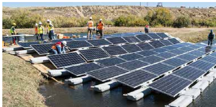
Floating Solar. FPV Installation in Walden, Co. Photo by Dennis Schroeder.
