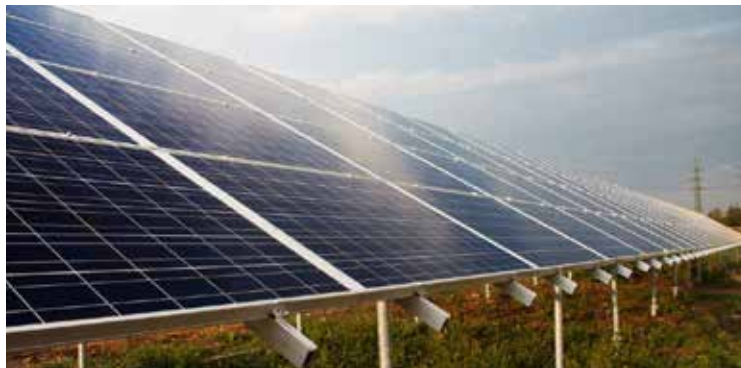
Ground Mount Solar PV System - stationary
