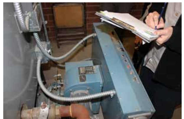
Recording nameplate information in a boiler room
