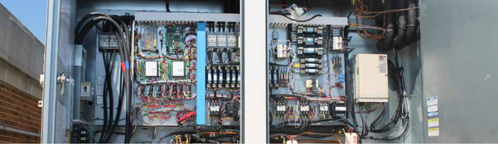
Internal controls of a high school Dedicated Outdoor Air Unit
