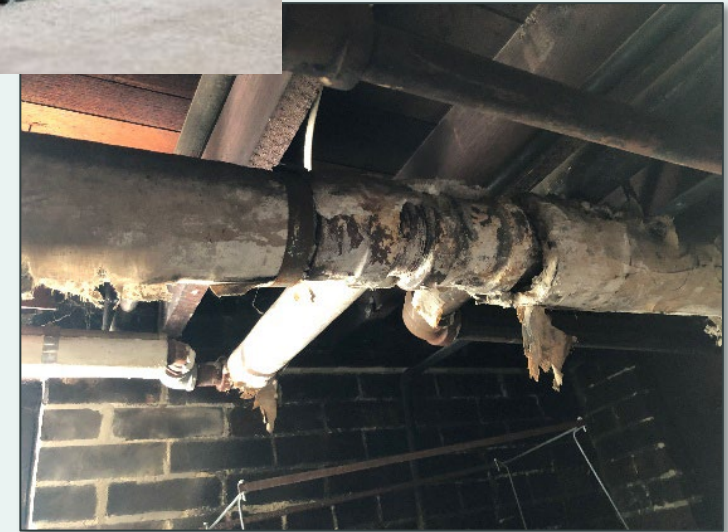
Asbestos pipe insulation
