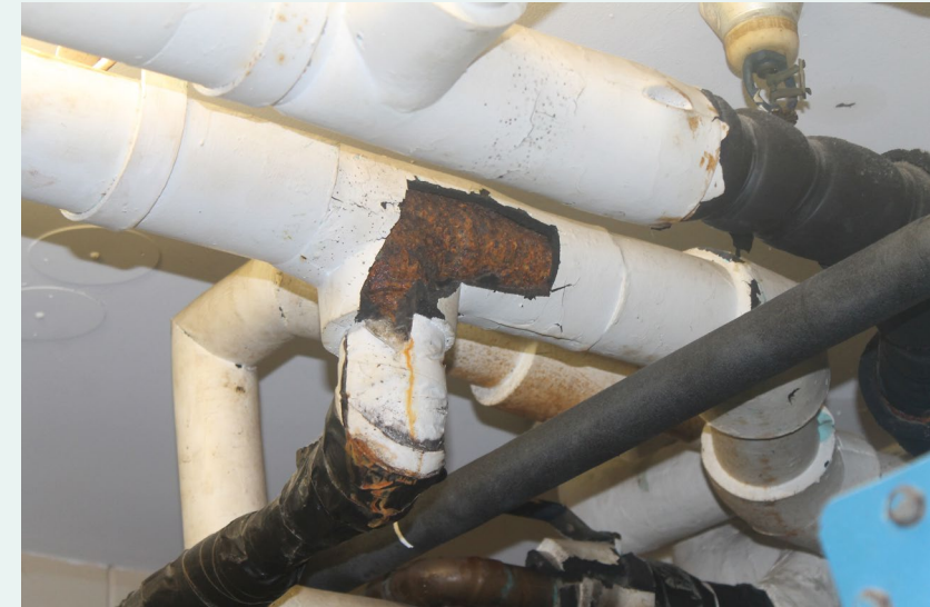
Corrosion Under Insulation (CUI)
