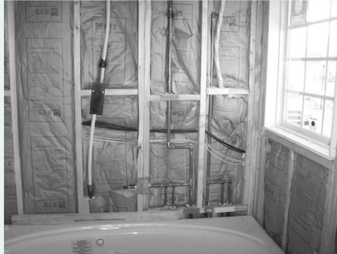
Uninsulated service water piping in wall cavities
