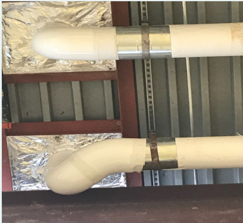
Poorly insulated downspouts
