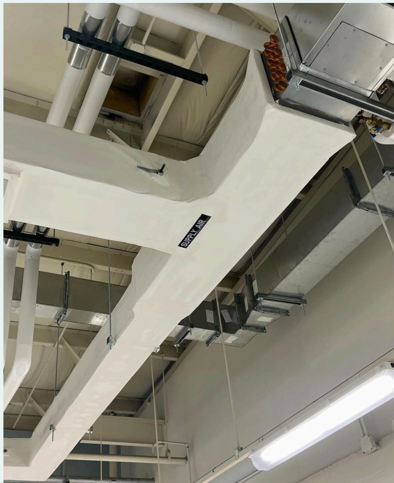
Properly sealed and supported duct insulation
