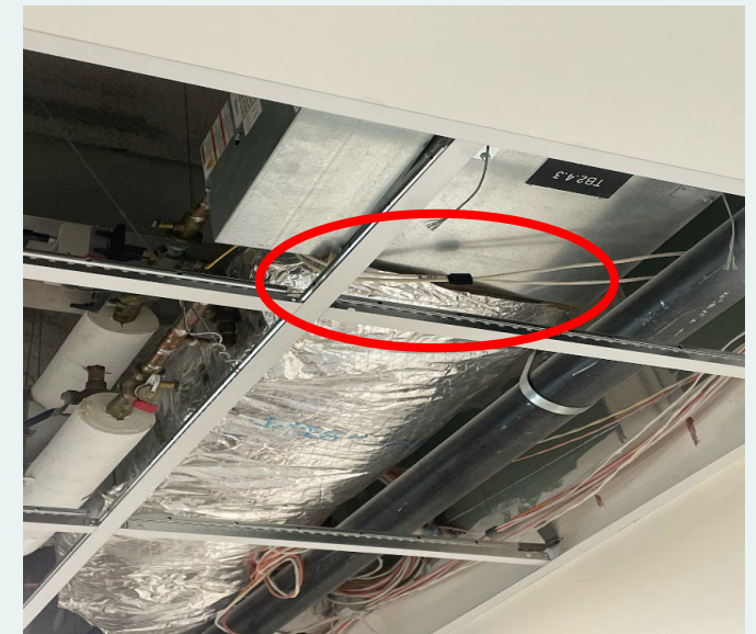
VAV box not taped
