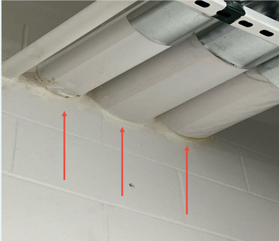
Insulation butts up to partition, but not continuous through assembly
