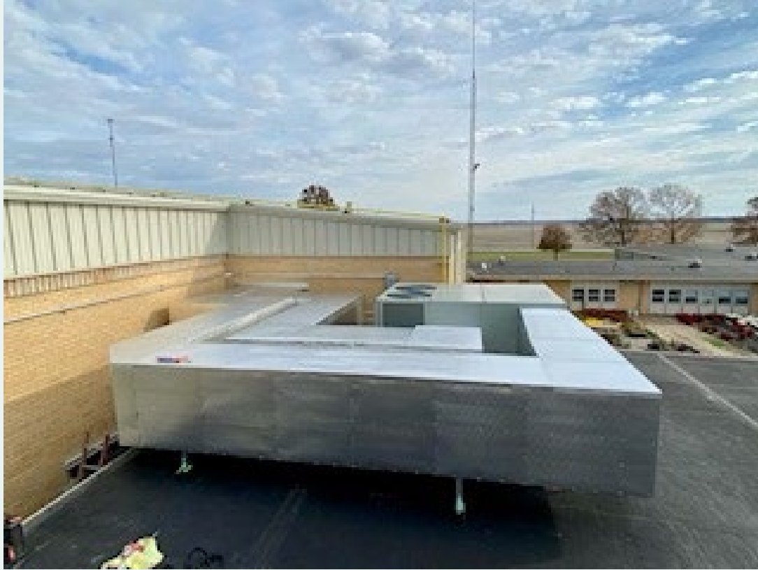
Insulated at proper temperatures
