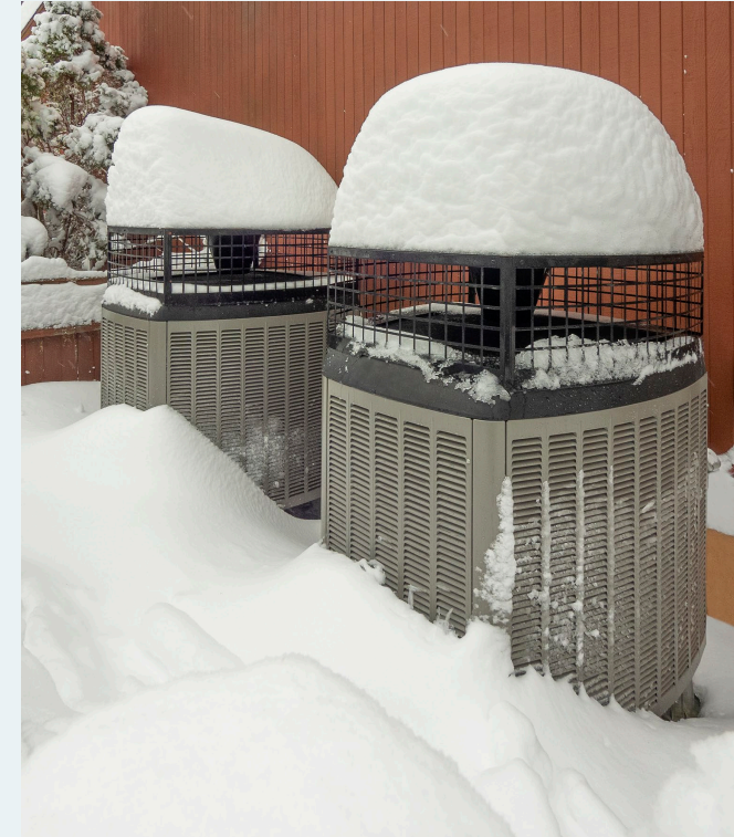
Air-source Heat Pump Condensers
