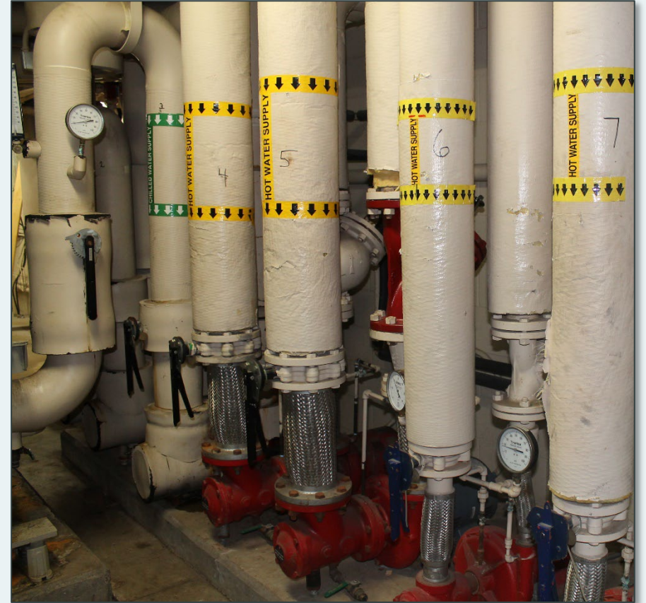
Typical install – SEDAC Assessment
