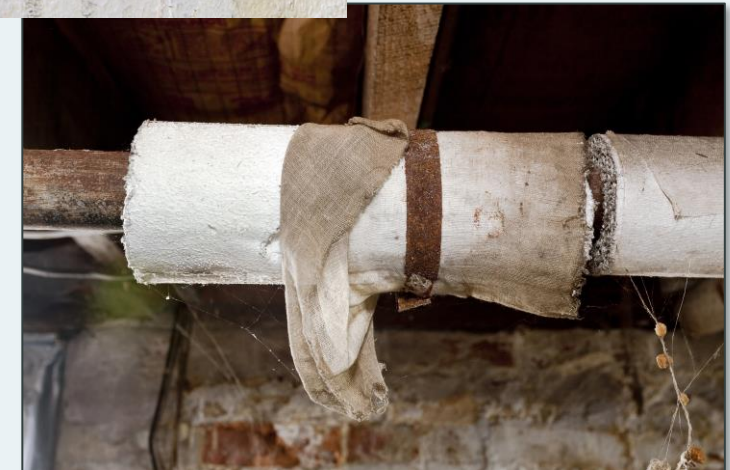
Asbestos pipe insulation
