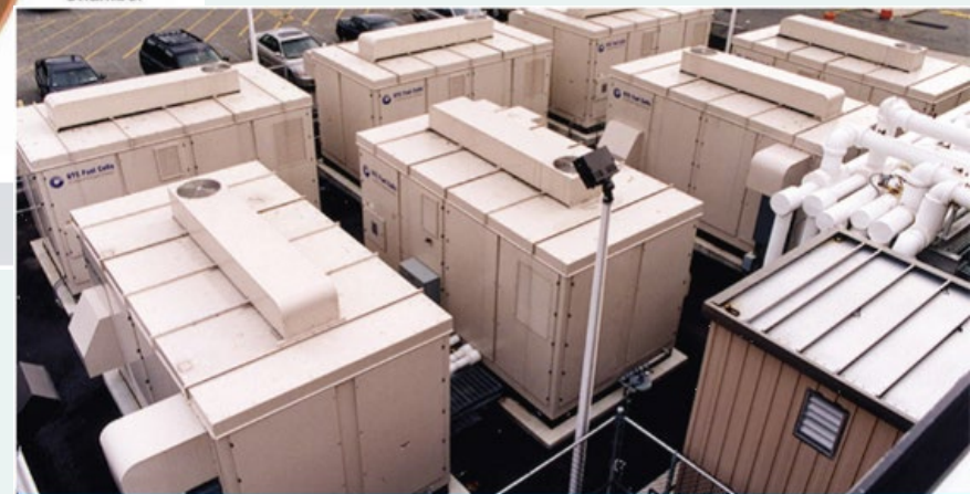
CHP fuel cell installation at Verizon data center. Photo courtesy of Verizon Communications.
