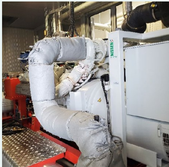
Reciprocating Engine at KWRD
