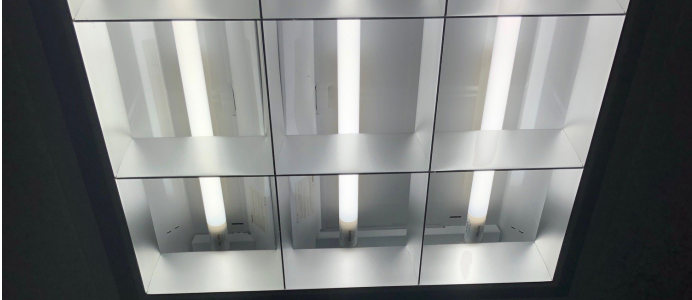
Linear LED retrofit lamps in existing fixture
